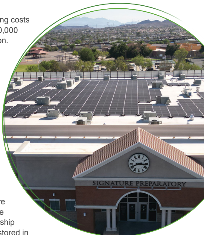
A 228-kW rooftop solar project atop the Signature Preparatory Charter School in Henderson, NV.
